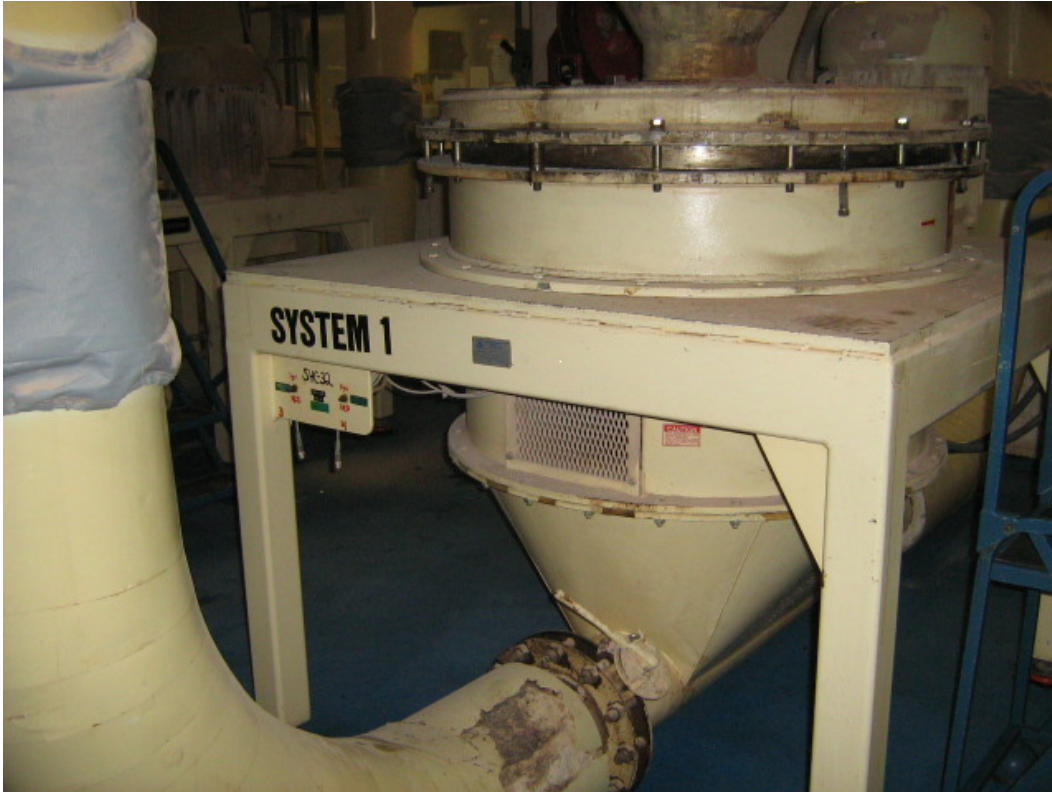
Figure 1: GM0001-L / 3C Grinding Mill #1.
